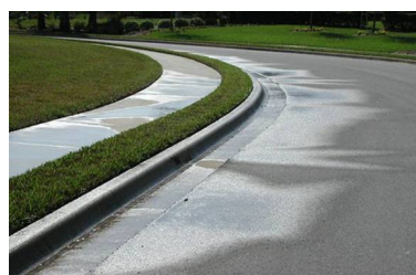
Figure 10. Irrigating this small strip of turfgrass with too large a spray head and excessive radial coverage results in water waste Credits: Michael Dukes
